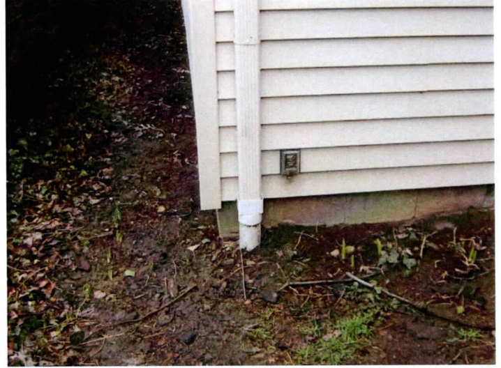
Improper Connection to Sanitary
